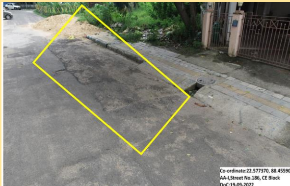
Drone used to identify road stretch in CE Block, AA I in New Town that required immediate attention of the authority
