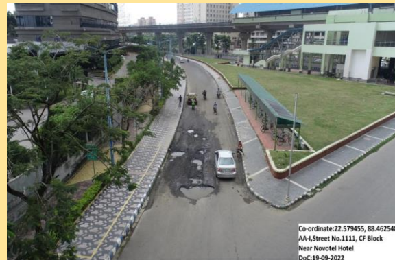
Drone used to identify road stretch near Novotel Hotel, AA I in New Town that required immediate attention of the authority
