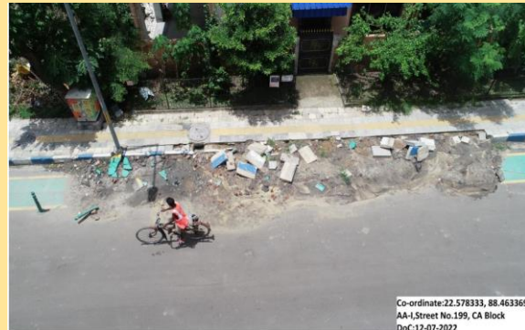
Damaged cycle tracks post installation of Gas Pipeline in CA Block, Action Area I
