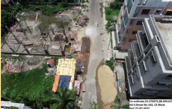
Drone Survey to identify dumping of construction materials in CE Block, Action Area I
