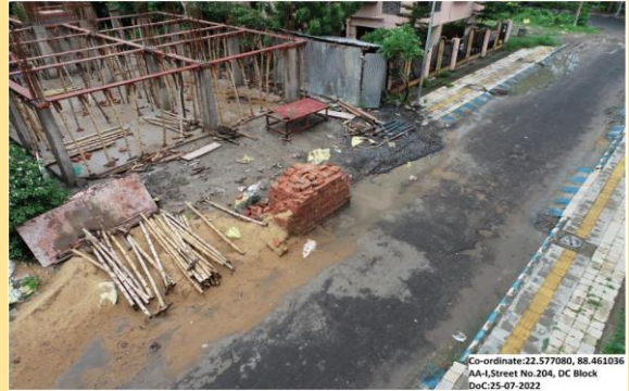
Drone Survey to identify dumping of construction materials in DC Block, Action Area I
